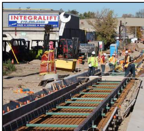
Laying of the southbound ION track on Borden Avenue. The camera is looking northeast from Bedford Rd. Note the track construction. A rebar mat is laid in the track trench. Vertical bolts that can be adjusted for height hold up tie bars on which rubber encased track has been placed. Concrete will then be poured from the rebar mat to the top of rail. Photo by Iain Hendry.
