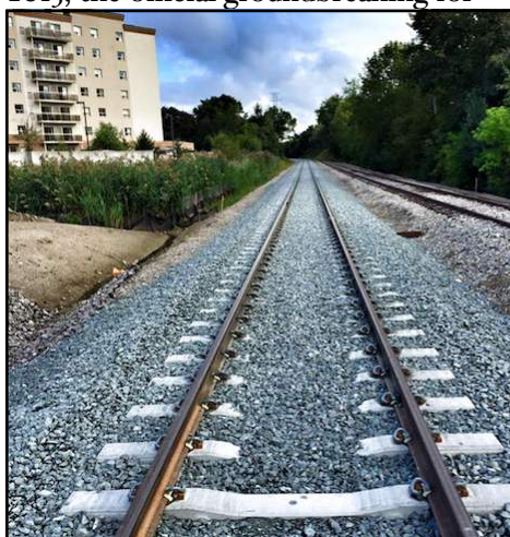
New double-track on Waterloo Spur awaiting electrification for the ION. Photo by Iain Hendry.
